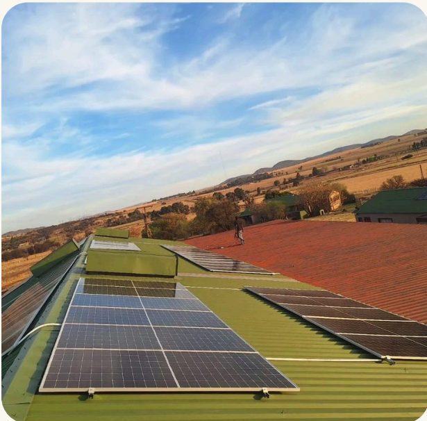
Commercial rooftop array
