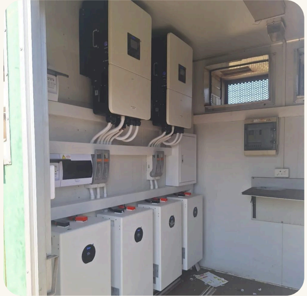
Inverter & battery room
