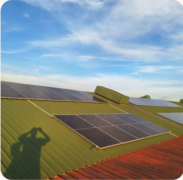
Roof-mounted PV array
